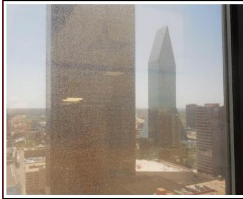
PHOTO #4. Failed IGU. Note the moisture stains at the interior of the airspace.
