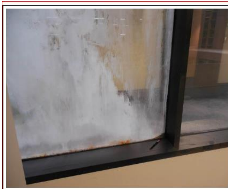
PHOTO #3. Failed IGU. Note the moisture stains at the interior of the airspace as well as the loose desiccant material outside the spacer at the lower right corner.
